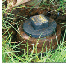
Cleanout sanitary sewer line access
